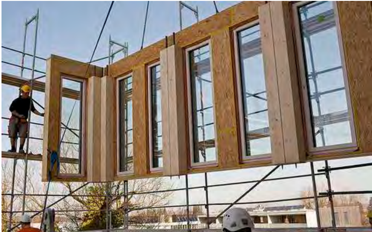
Figure 17: Wood Hybrid Modular System at Life Cycle Tower One (LCT One), Austria, 2012
